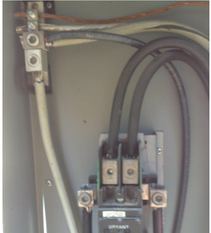
Main Breaker Panel
