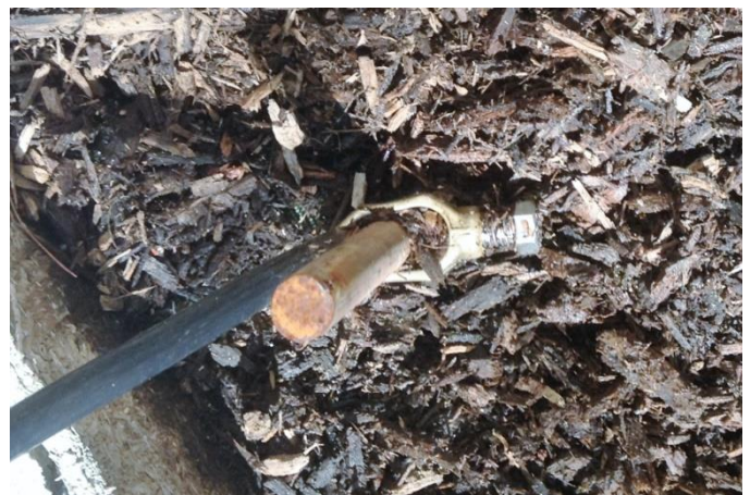
Ground rod, cable, and clamp ke8cqw photo
